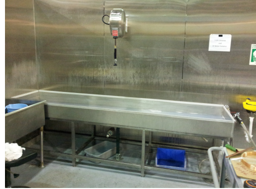
Figure 30: Pre Cleaning station.
